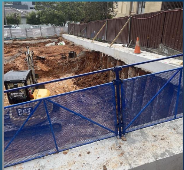
Building Pit Protection 1.2m high
